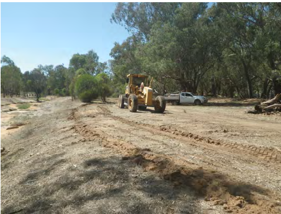
Left: Fire Mitigation Services (FMS) grader working along Boyagerring Brook. Works are not only reducing the fire hazard but allow scope for revegetation, public open space and passive recreation, including an extension to the popular 'Murray Walkway'.
